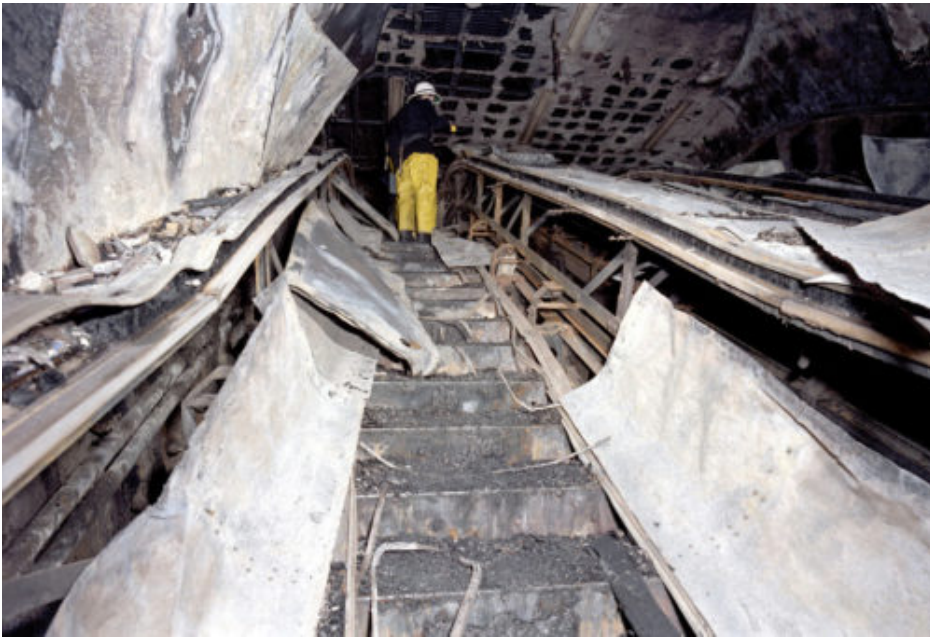
Wooden escalator after the fire. Copyright The London Fire Brigade
